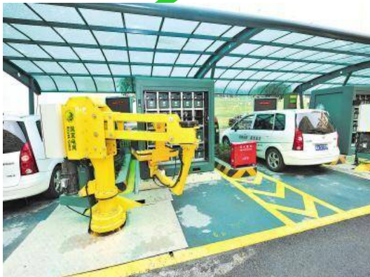
Charging and Swap station
