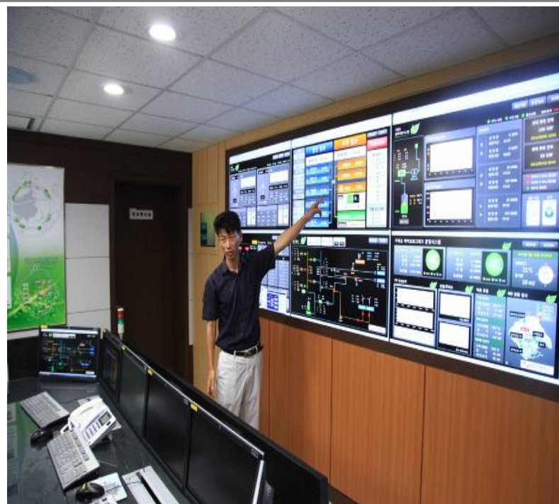
Integrated Micro Grid Operation Center
